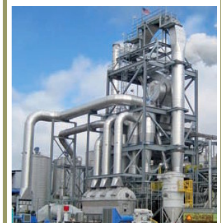
Ring Dryer Systems
